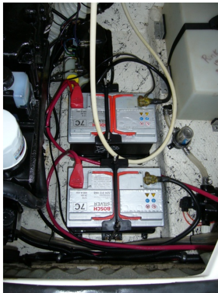
Figure 5 - Batteries in a motor boat.
