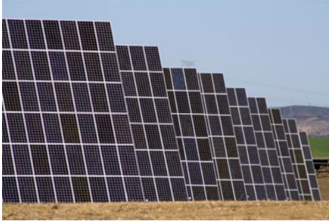
Fig. 9. Casaquemada PV plant (Solucar Platform, Sanlucar la Mayor, Seville, Spain).
