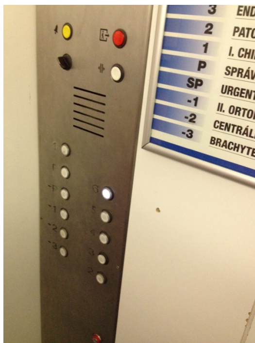
Figure 15: Lift buttons and signs at FN Motol
