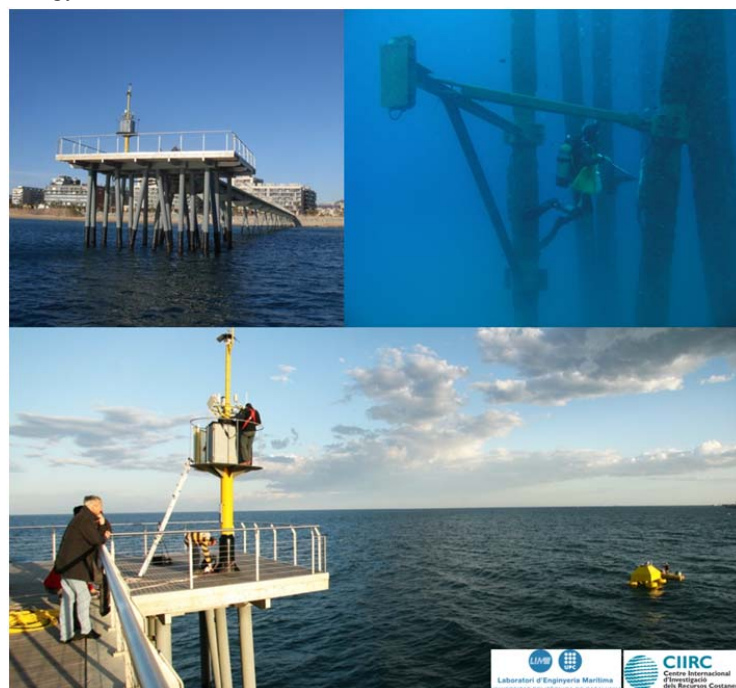
Figure 4. Sample illustrations of the instrumented coastal pier scientifically managed by UPC in Barcelona and located off the Badalona coast. The upper left panel shows an overall picture of the pier type (at a water depth of about 13m) while the upper right and lower panel illustrate the deployment of observational equipment in one of the legs and for the testing of a floating buoy.
