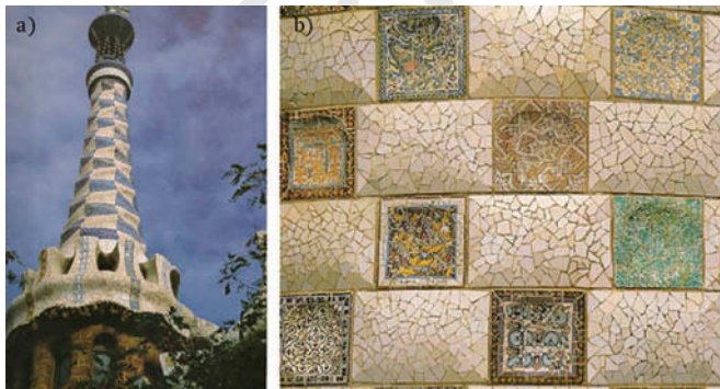
FIG. 4. (a) Roof the Parque Güell entrance hall, and (b) precast elements of the side walls of the main stairway. © (a) J. Bergós. Reproduced by permission of (a) J. Bergós. Permission to reuse must be obtained from the rightsholder.
