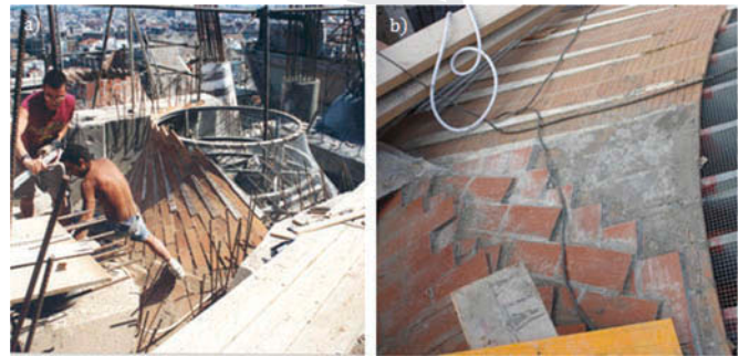
FIG. 19. (a) Construction process of the hyperboloids of the building, and (b) detail of the triangular pieces positioned between the ceramic pieces (ATESF).
