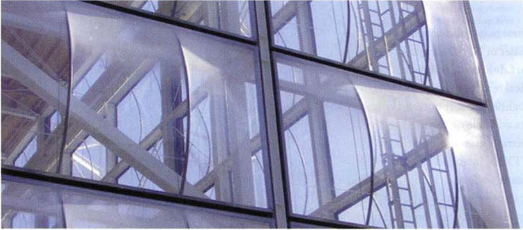
Fig. 11. Bergwatch Bayern training center, Hightex. Fig. 11. Centro de Entrenamiento de Bergwatch Bayern, Hightex.
