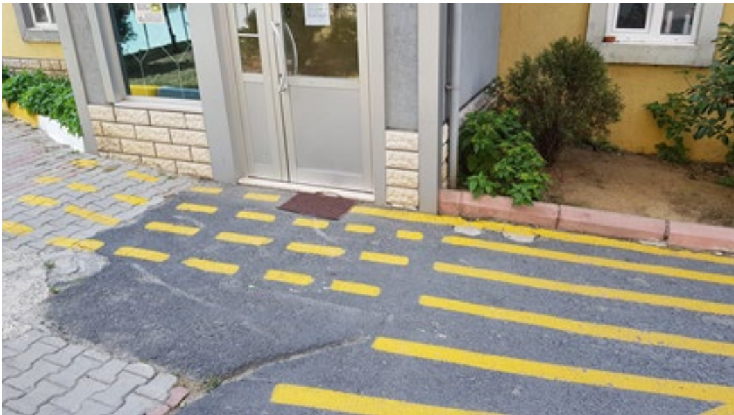
Figure 1. Building entrance with inadequate design for access
