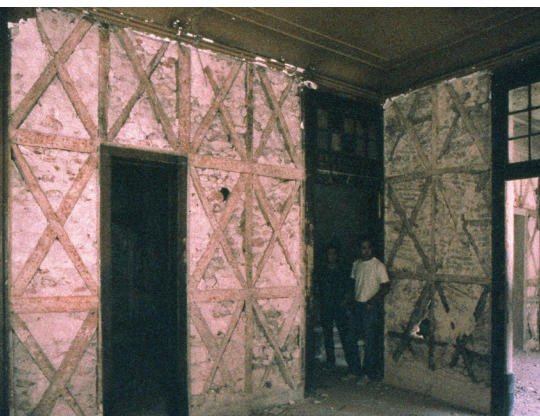
How can another earthquake such as that of Lisbon be withstood? Building in Rua Augusta, 82-84, Lisbon. © Ramon Graus, 1992.
