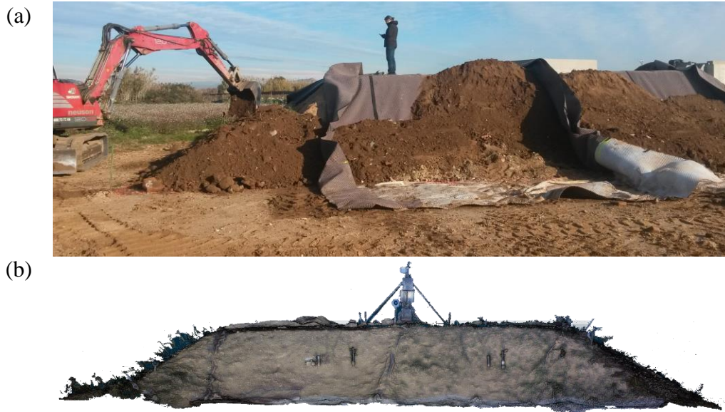
Figure 2.1: (a) Photograph of the embankment during the construction. ; (b) 3D view of the point cloud obtained by terrestrial laser scanning.
