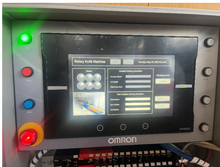
Figure 5.2.6. Main HMI screen (source: own).
