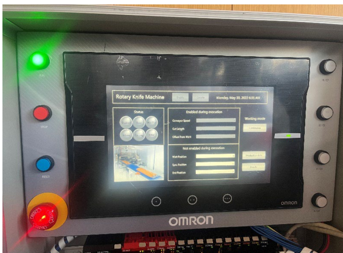
Figure 5.1.9. Main HMI screen (source: own).
