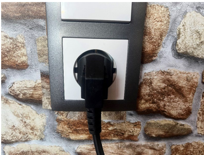
Figure 5.1.1. Connecting demo case power cable to 230 V (source: own).
