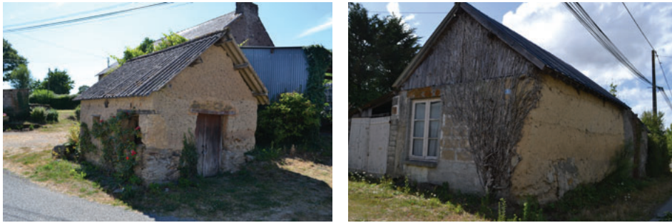
Fig. 02. Examples of raw earth constructions in the Fégréac and Chevallerais cities ©M. Miranda
