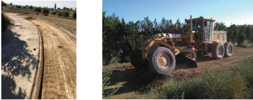
Figure 2. Milling procedure of the original surface and levelling process of the borrow soil.
