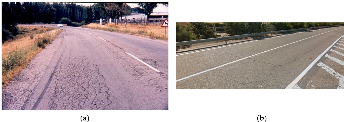
Figure 13. (a) Cracks from the top down and (b) Typical alligator skin cracking failure.
