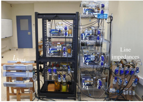
Fig. 6. Photograph of the experimental microgrid.
