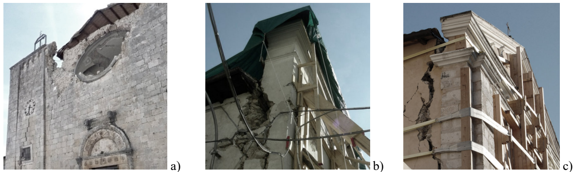
Figure 1: Partial collapses observed in the Italian churches of Sant'Eusanio Martire in Sant'Eusanio Forconese (a), Santa Maria degli Angeli in Paganica (b) and Santa Gemma in Goriano Sicoli (c) (L'Aquila district, Abruzzi).
