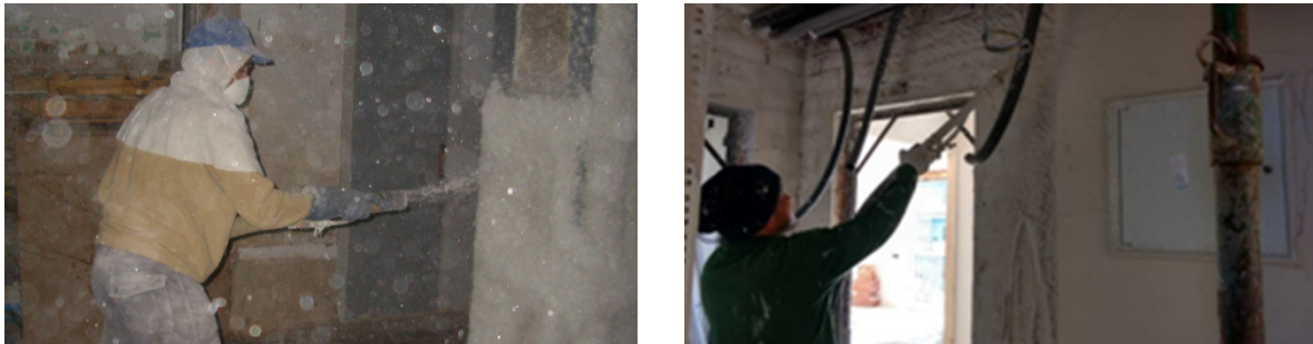
Fig. 1: Methods of applying building products to a vertical surface using a sprayer. Left: mortar cement. Right: gypsum plaster Source: authors
