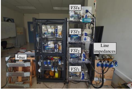
Fig. 3. Photograph of the experimental microgrid.
