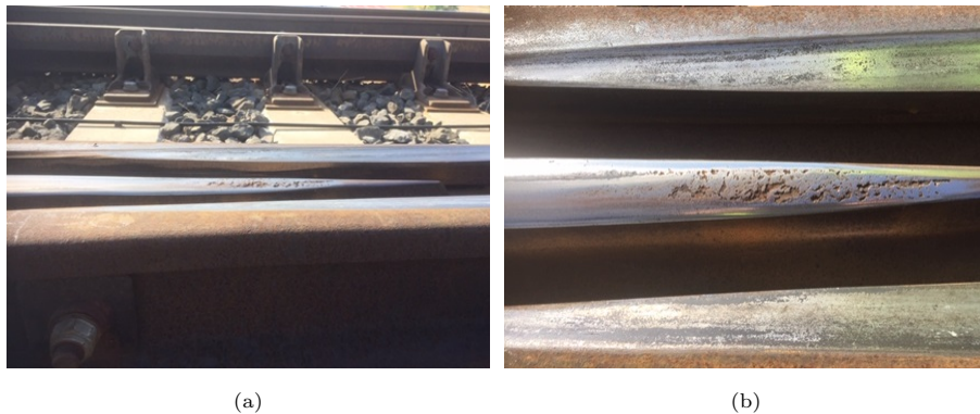
Figure 2: Fatigue degradation detected at the frog nose element placed at the Puertollano line. a) General and b) detail views. Source: CIMNE.
