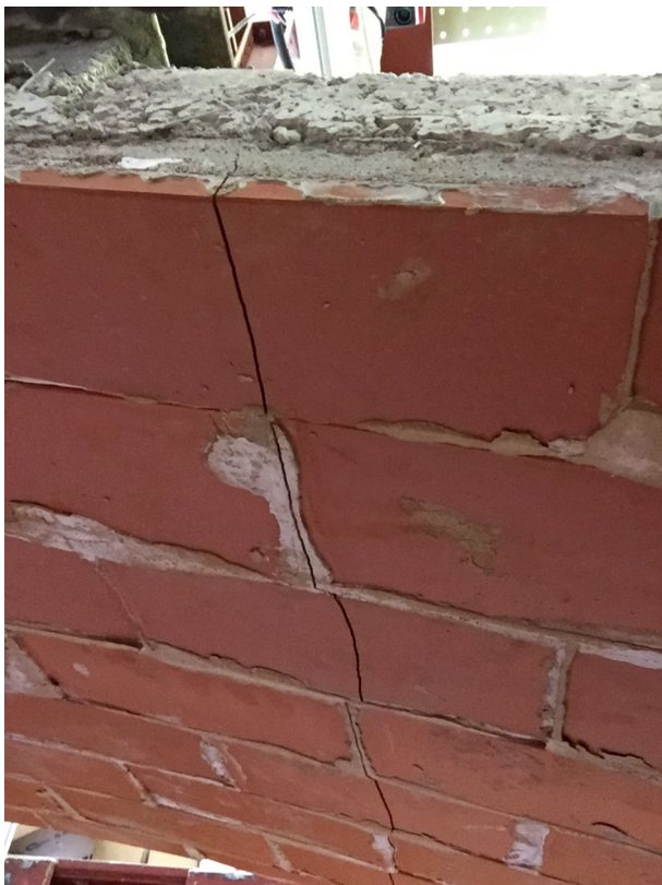
Fig. 10. Crack on the intrados of the composite barrel vault 1 showing the formation of the first hinge.
