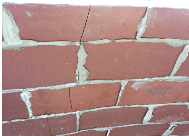
Fig. 11. Cracks on the intrados of the composite barrel vault 2 showing the formation of the first hinge.
