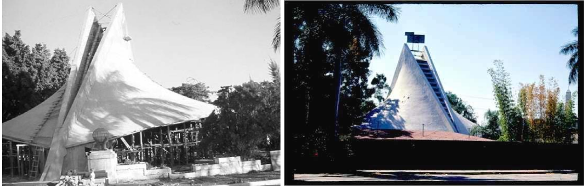
Figure 20. Construction of the hyperbolic paraboloid (left) and external view of the discoteques (right) in Hotel Casino de la Selva.
