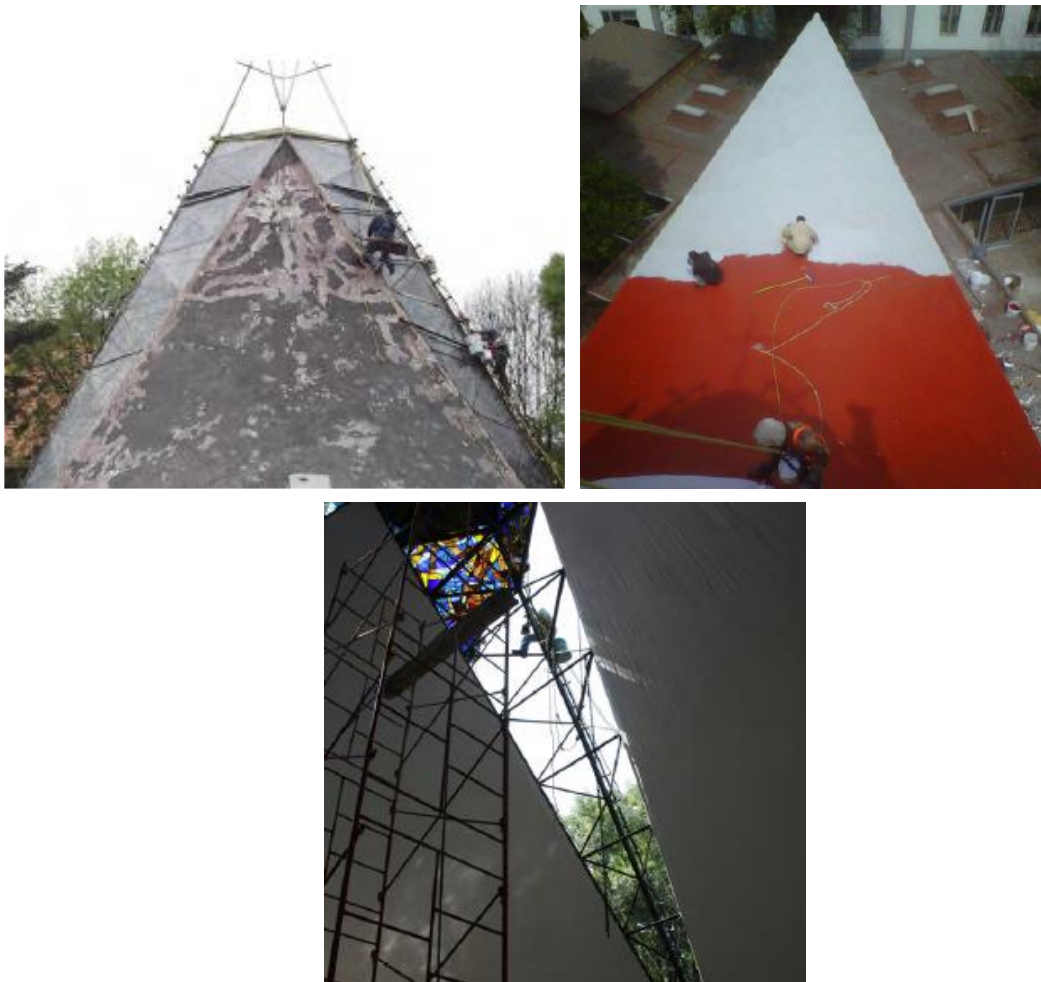
Figure 44. Crack injections (left), waterproof and paint coating application (right), and corrosion cleaning (bottom) at San Vicente de Paul.
