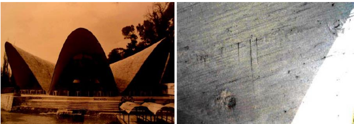
Figure 38. Shrinkage cracks pattern after construction (left) and patched leaks (right) in Los Manantiales.
