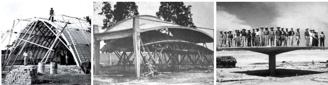
Figure 12. Experimental models: funicular vault in San Bartolo (left), Fernández factory (center) Inverted umbrella (right).
