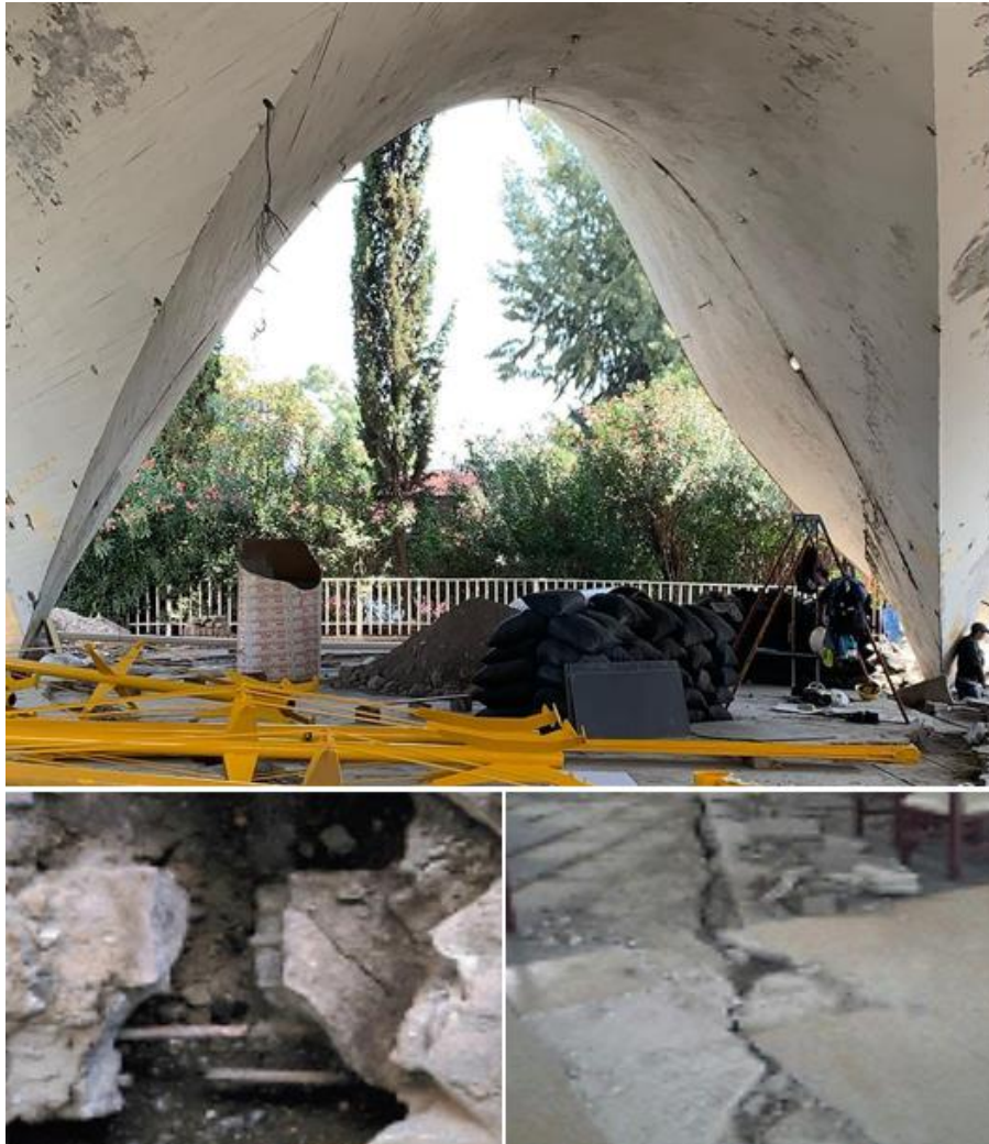
Figure 41. Lost of geometry at the hypar of Los Manantiales (top), Broke tie (left), and ground fracture (right).
