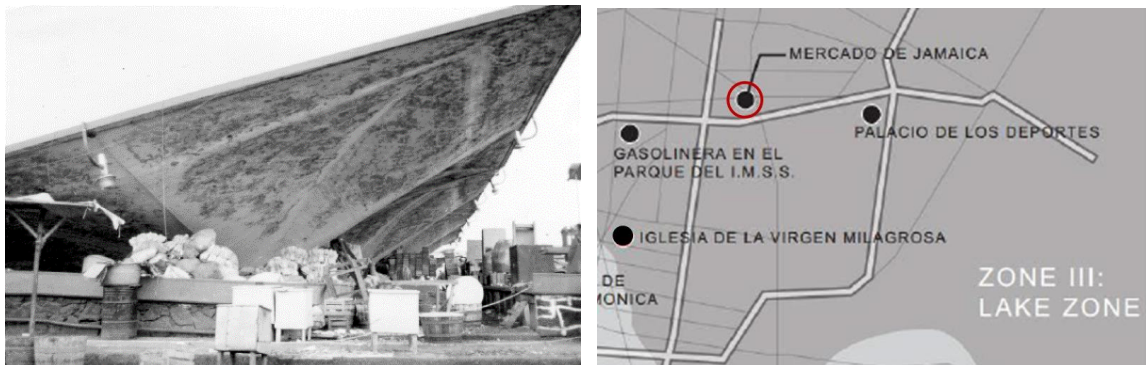
Figure 23. Collapse of umbrella columns, shells are seen without apparent noticeable damage (left) and location and soil types in Mexico City (right).
