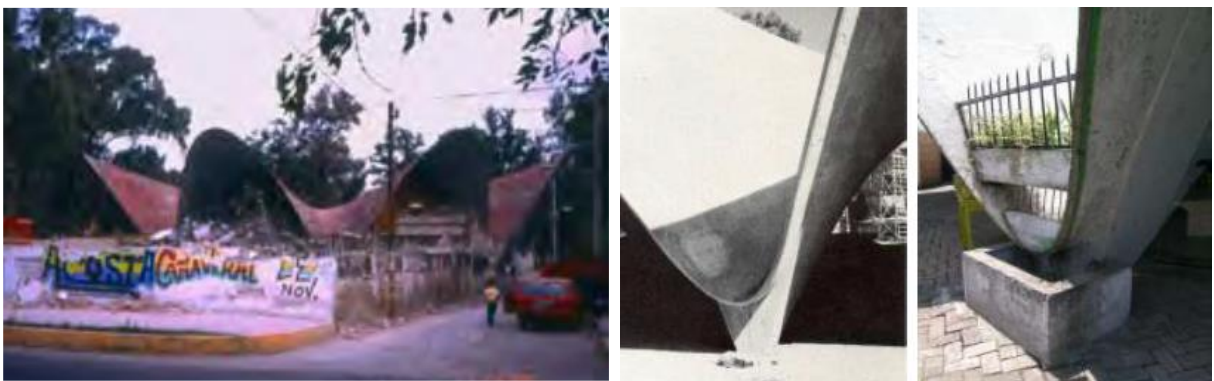
Figure 40. Red waterproofing in 1996 (left) and protections and addition of water collector (center and right).
