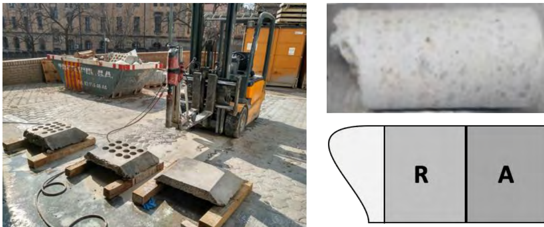
Figure 1. Extraction of sprayed concrete specimens (a) and division of samples into part A and part B.
