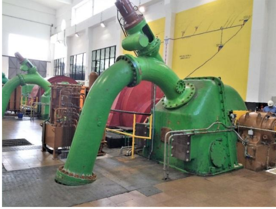
Figure 18. View of the Pelton unit 2
