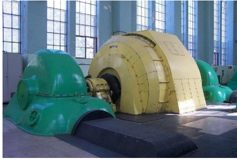
Figure 2. View of the Pelton unit
