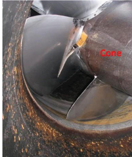
Figure 2: Crack found in one blade of a bulb turbine unit
