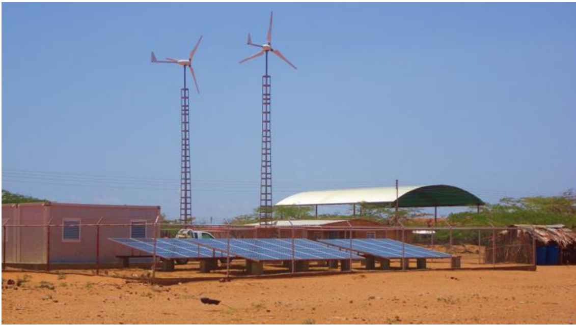
Figure 2. Hybrid microgrid and school in the community of Cúsia
