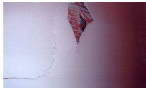
Figure 22 – view detail photo of cracking in the walls of masonry of ceramic pieces in an apartment building
