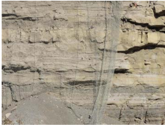
Figure 1: Application of double-twisted hexagonal rockfall mesh in a mine in New South Wales, Australia.
