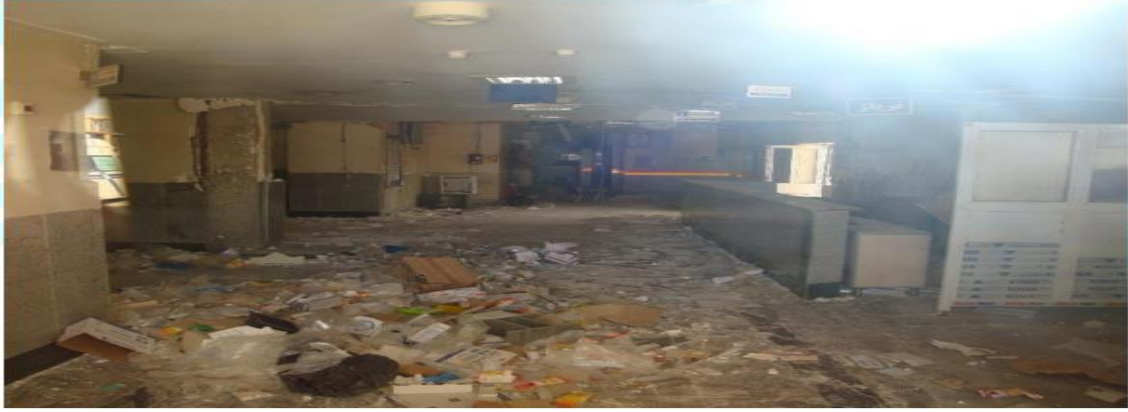
Figure. 3.13. Severe injuries to Sarpol-e Zahab martyrs hospital (Kalantari, 2017).
