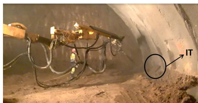
Figure 17. Concrete projection for the tunnel construction of the B-40 in Viladecavalls (Barcelona, Spain). For that purpose, 3 different ITs were tested during three different projections of recycled concrete to monitor the first 40 hours of curing, Figure 18a. In Figure 18b the positions of the transducer on each IT can be seen.
