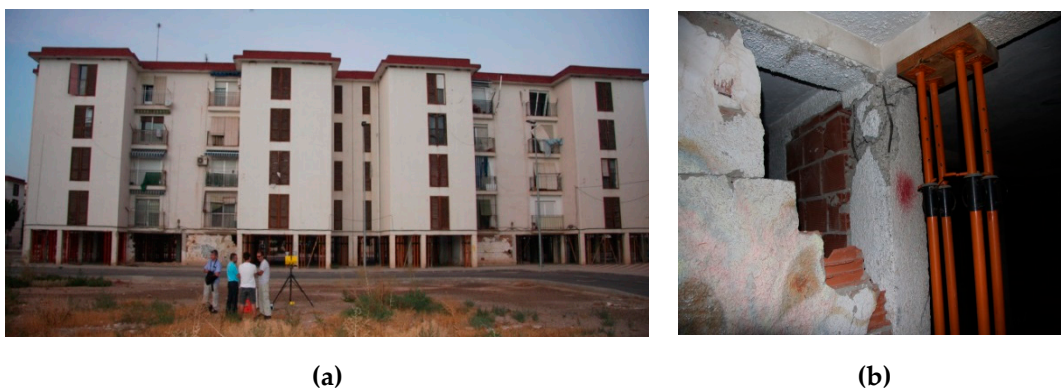
Figure 3. (a) Typical buildings in San Fernando neighbourhood; (b) Example of a damaged pillar.
