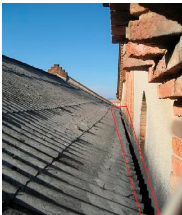
Figure 22. Dampness in the joint between the roof and the façade.
