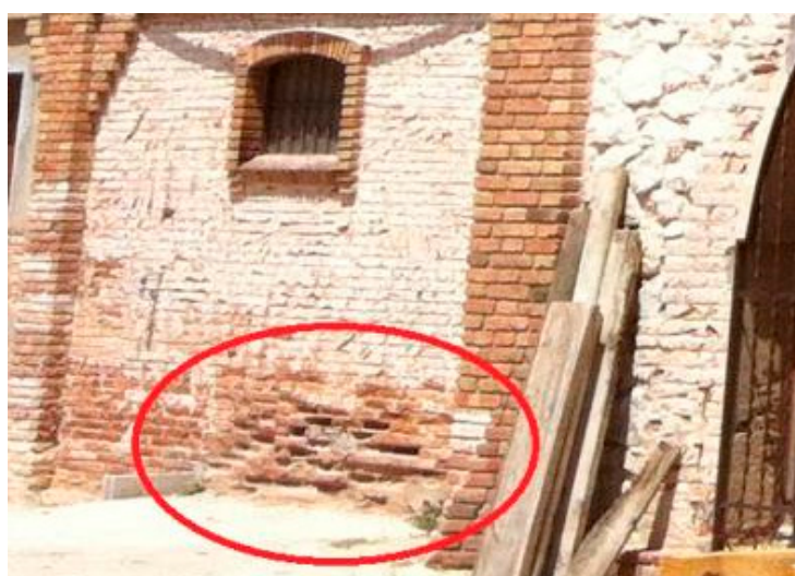
Figure 13. Deterioration of the base of the façade.
