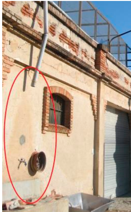
Figure 15. Dampness on the façade.
