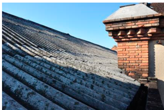
Figure 21. Condition of the roof of the wine-production nave (exterior) before restoration.
