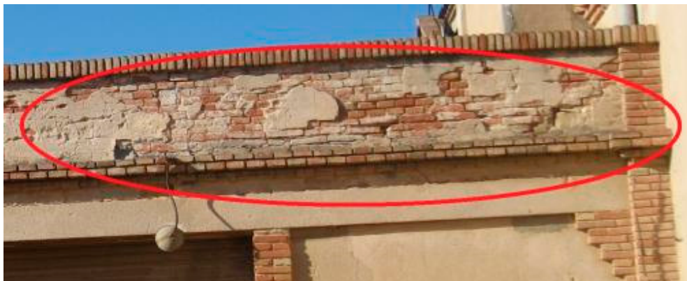
Figure 11. Loose render on the walls of the façade.
