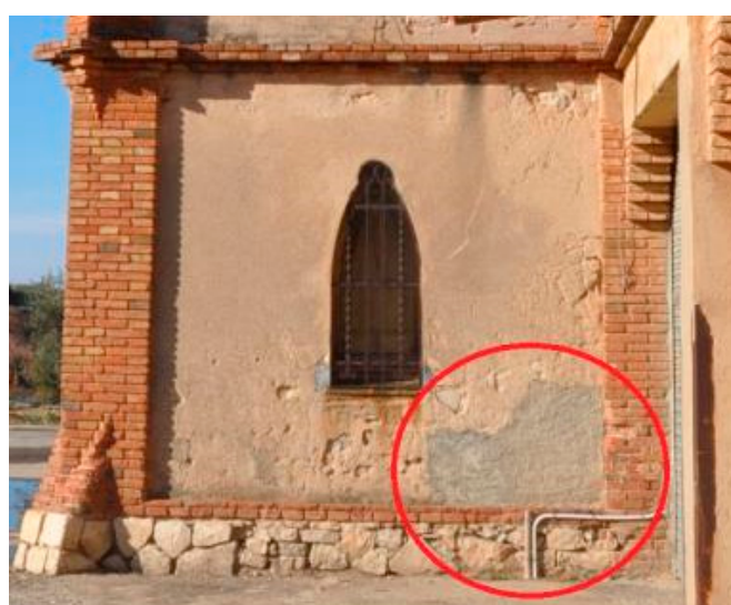
Figure 14. Addition of material that was not original to the façade.
