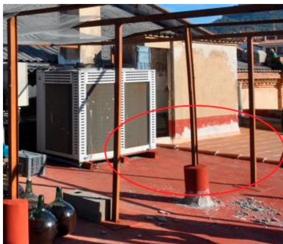
Figure 20. Discordant paving on the flat roof.
