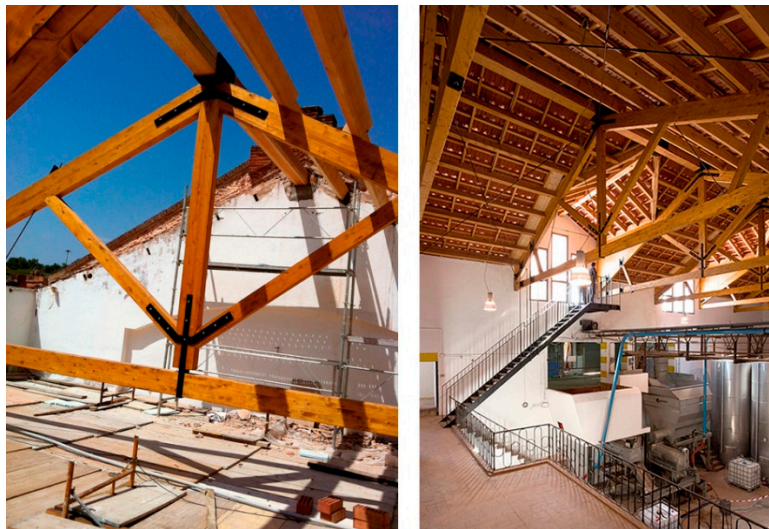
Figure 27. Roof structure of the wine-production nave during restoration ( left ). Roof structure of the wine-production nave after restoration ( right ).
