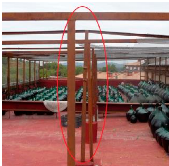
Figure 17. Rusting of metal structures on the flat roof.
