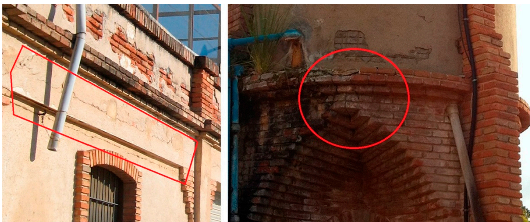
Figure 16. Cracks in the top part of the façade and in the water tank.
