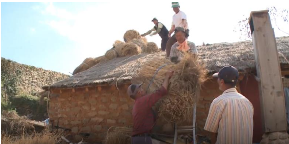
Figure 53: Replacing of the straw covering in the roof of Choga in Nak-an, Korea [49]
