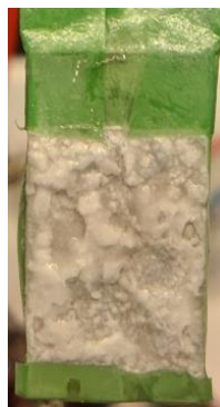
Figure 54. Bare aluminum plate corrosion.
