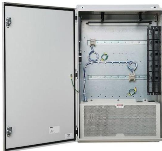
Figure 8.31- Electrical cupboard for the components' distribution. Source [19].
