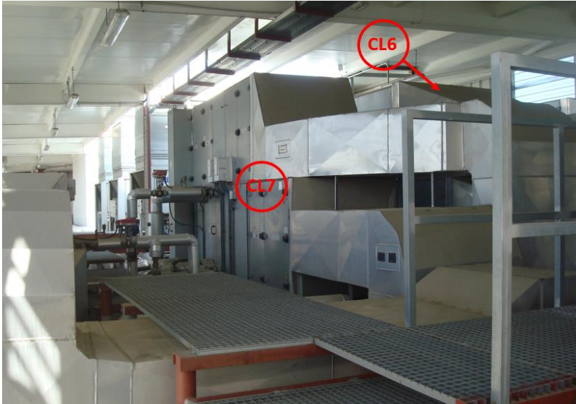
Figure 63: Zone located on the right side of the TBS zone where the AHU's CL5, 6, 7 and 8 are located
