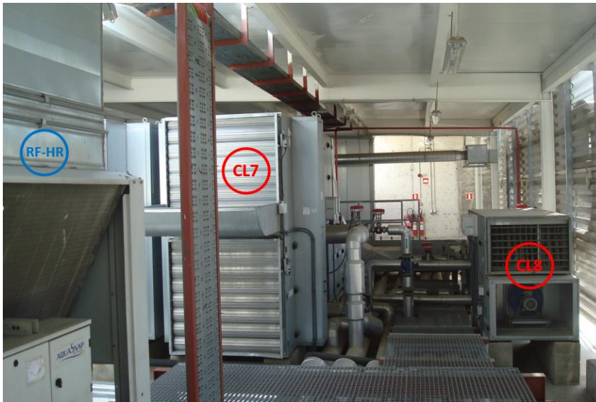
Figure 62: Detail of the RF-HR cooling tower, and AHU's CL7 and CL8
