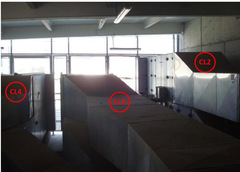
Figure 64: Zone located on the left side of the TBS zone where the AHU's CL1, 2, 3 and 4 are located
