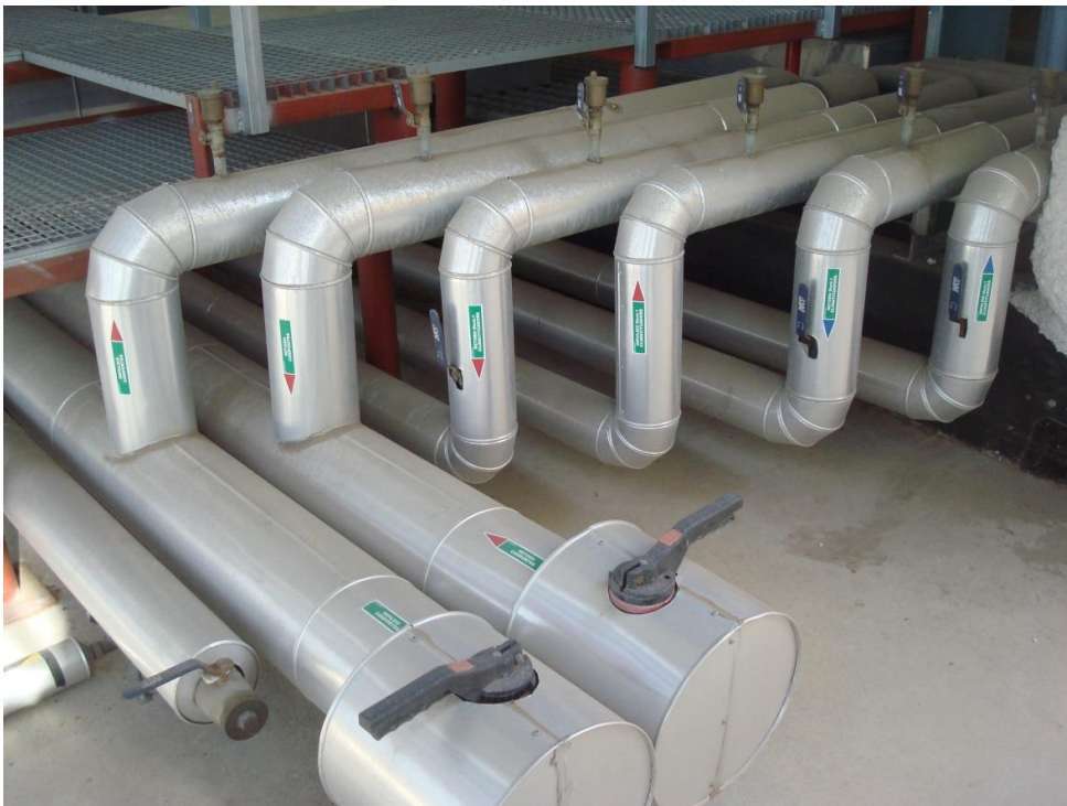
Figure 60: Detail of the distribution of hot and cold water pipes
