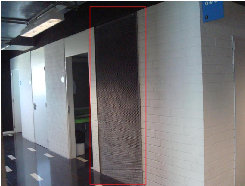
Figure 59: General extraction grille located on a corridor
