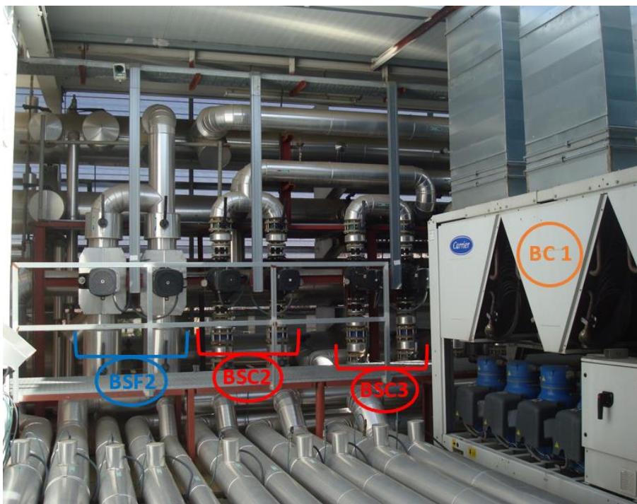
Figure 57: Secondary circuit pumps together with heat pump BC1
