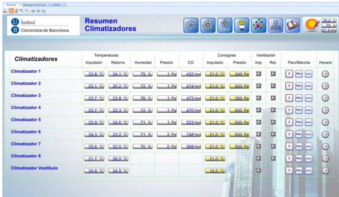
Figure 61: Air Handling Units control display
