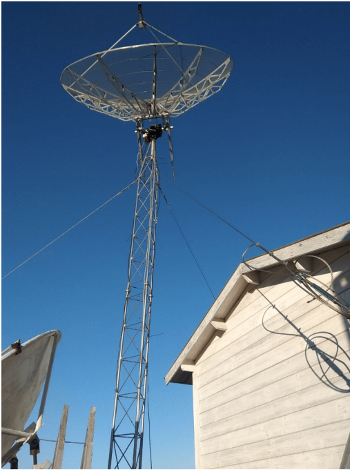
(a) Finished antenna
