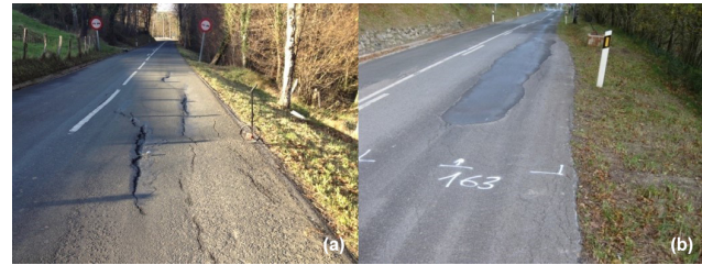
Figure 9. Road sections situated within slow-moving landslides with damage shown: (a) PoR C3C of the road GI-2133 (from km 8.280) with observed deformations and cracks on the road pavement; (b) PoR C9G of the road GI-2637 (from km 17.891 to 18.220) showing minor cracks already sealed.
