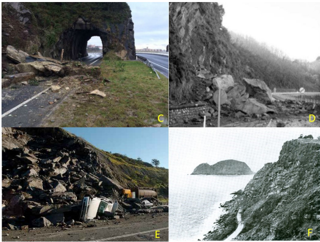
Figure 3. Examples of rockfall magnitudes (C, D, E, F) in the study area in relation to the classes of Table 2 (source: magnitudes C, D, E; Javi Colmenero; F, Servicio Geológico de Obras Públicas).
