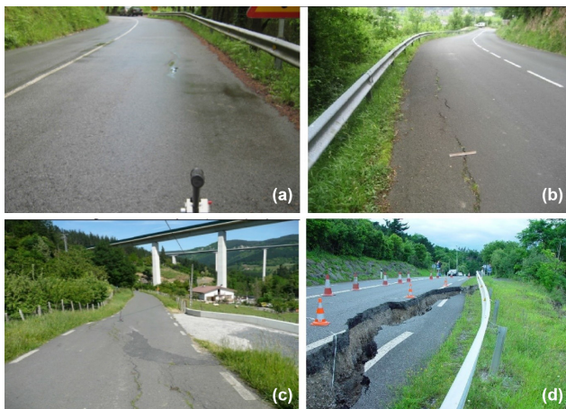
Figure 5. The four damage levels identified on the roads of Gipuzkoa: (a) no/slight damage, (b) moderate damage, (c) severe damage, and (d) partial/total destruction.
