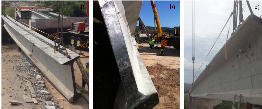
Figure 3. First lifting operation (a), deformed shape after first lifting (b) and deformed shape once in place after second lifting (c).
