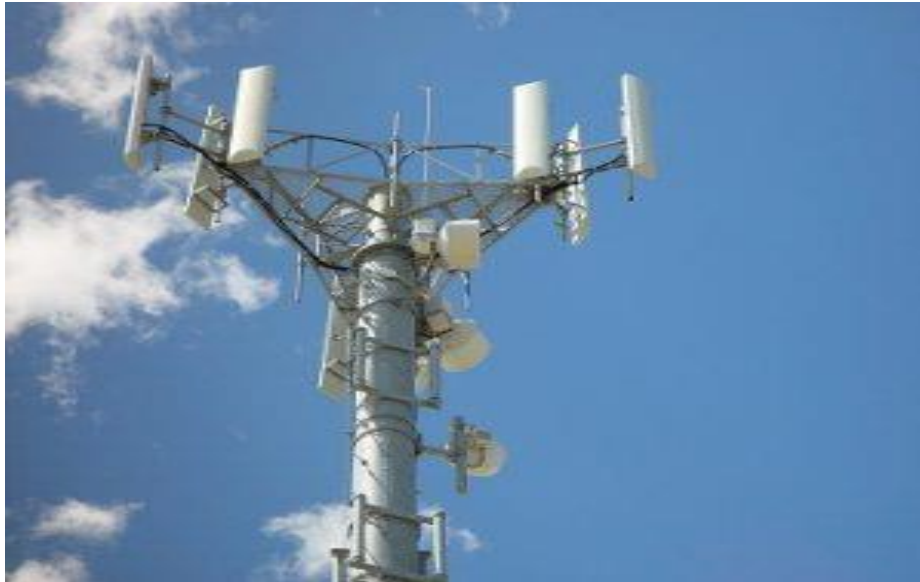
Figure 3.1.2-2 LTE base station
