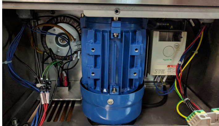
Figure 81. Interior of the electrical cabinet (1). Source: Own
