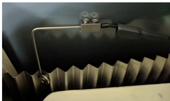
Figure 98. Connection inside the working tank between the cathode and the negative wire. Source: Own
