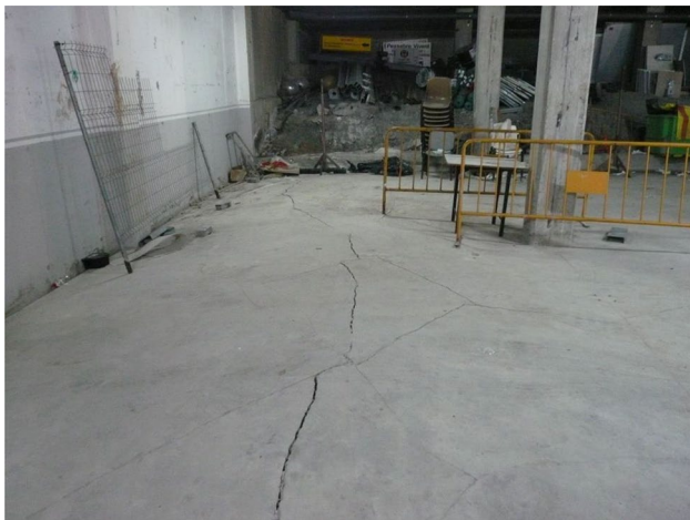
Fig. 2 Cracks and heave of the basement floor
