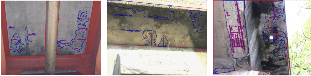
Figure 2: Sample images containing the ROI (red), delamination damage (blue), rebar exposure (purple) and non-damage regions.
