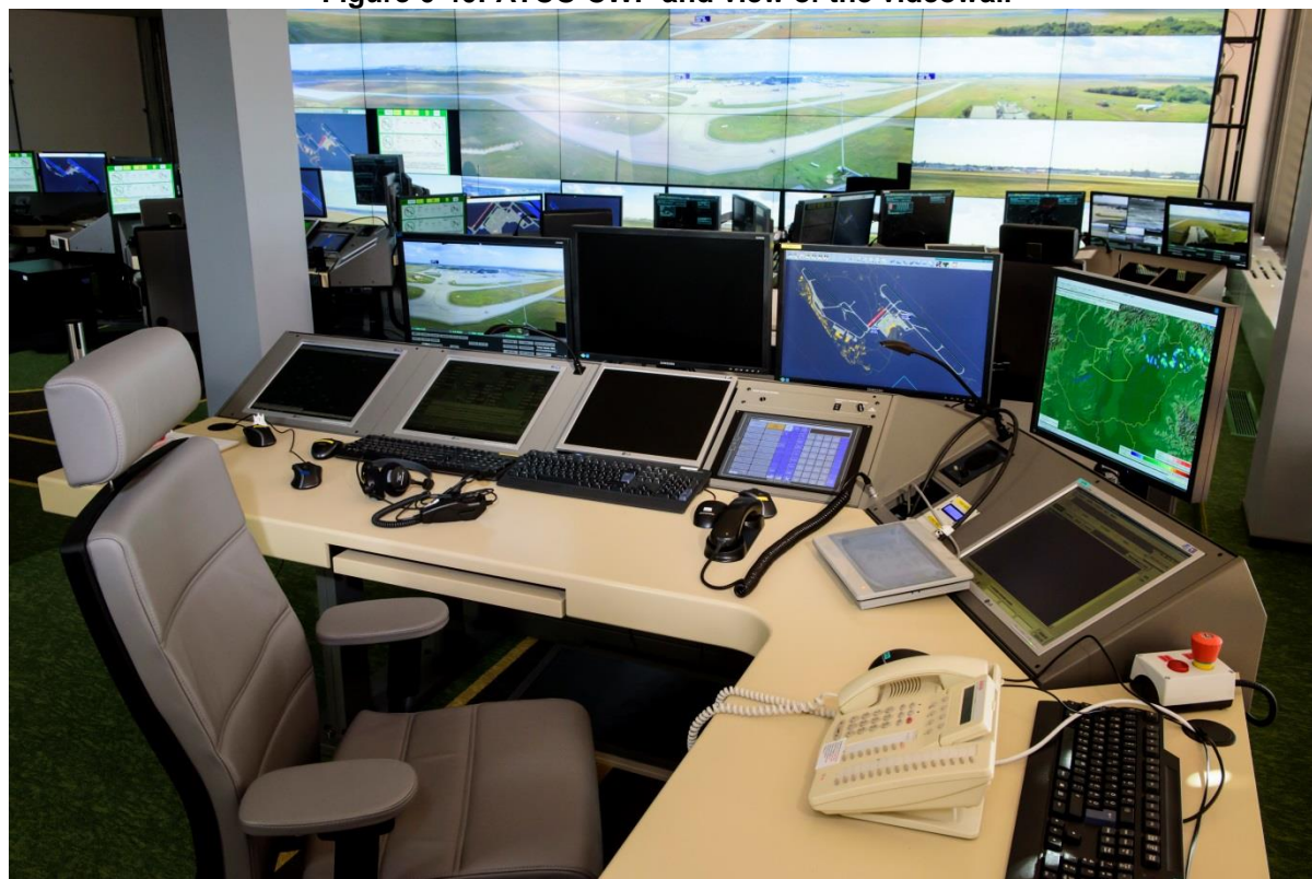
Figure 6-41: Supervisor position with videowall in the background
