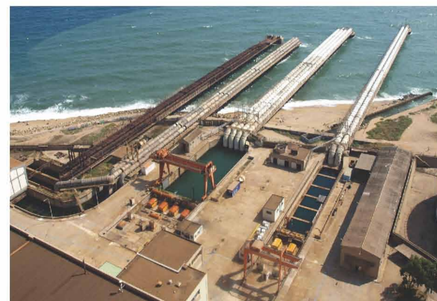
Water treatment system
