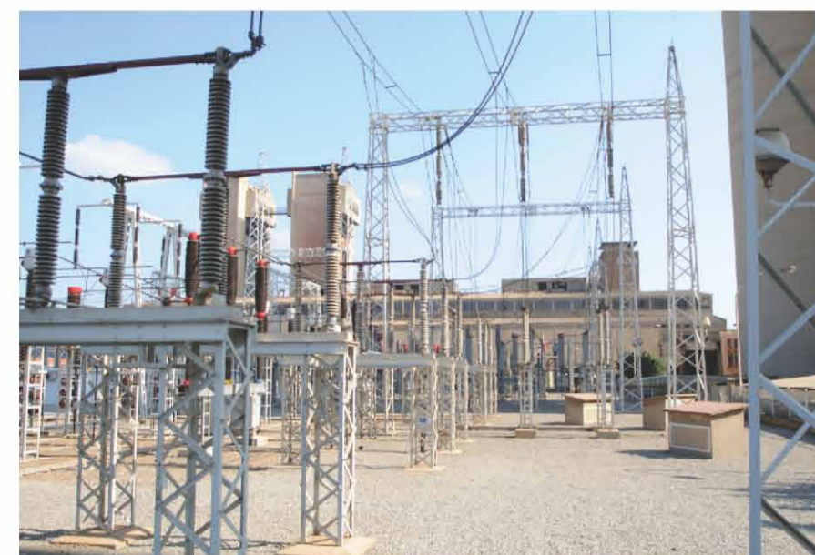
Immovable transformer central
