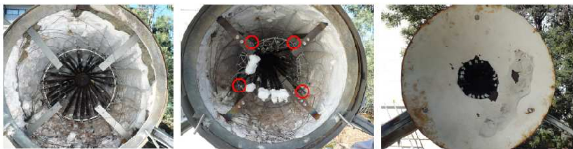
Figure 38. Three receiver configurations viewed looking in to the aperture. Left: Receiver with a 7.5° half cone angle (front shield removed). The indents in the wall insulation indicate the position of the tubes in the frustum with a 17.° half cone angle. Centre: Receiver in a frustum with base radius 77 mm (front shield removed). Right: Receiver as a frustum with base radius 77 mm, but with minimal insulation on feeder tubes (front shield in place).
