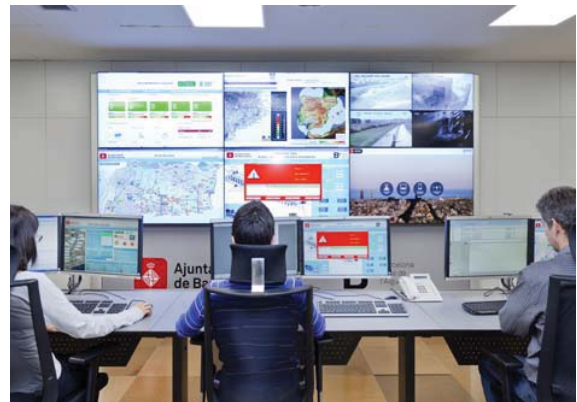
Fig. 6. Control center for Barcelona sewage network. Courtesy of BCASA company [5].
