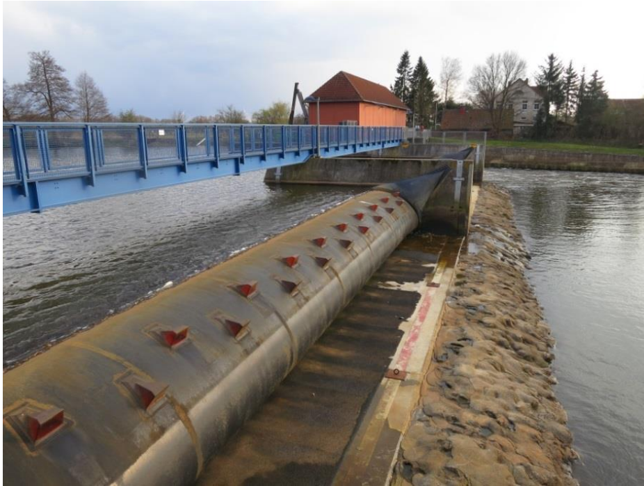
Figure 1: Inflatable dam with breakers near Marklendorf at the river Aller
