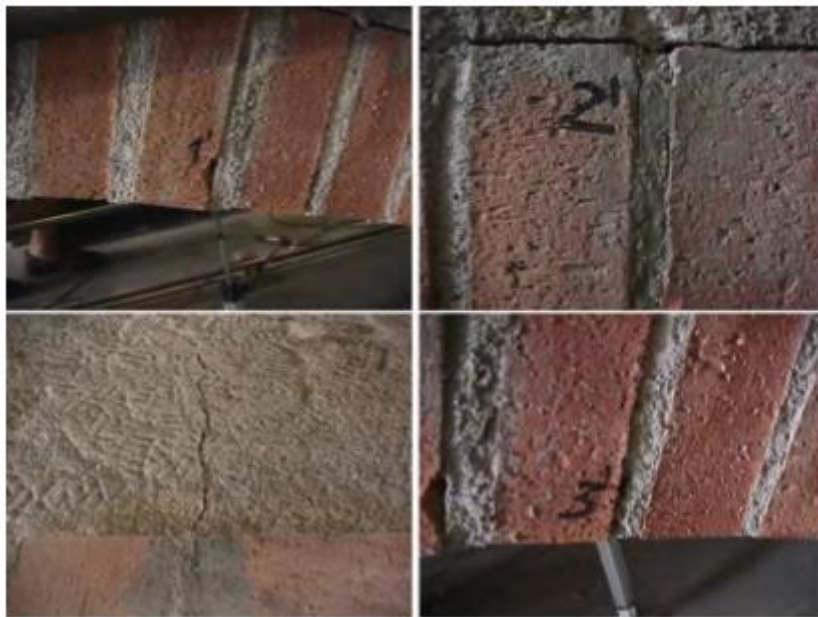
Figure 3-18 cracks in the east side for a load below 5 tons (Serna, J., 2001).
