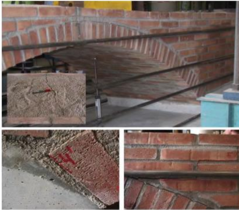
Figure 3-19 general view of the east side and some cracks just before the collapse (Serna, J., 2001).
