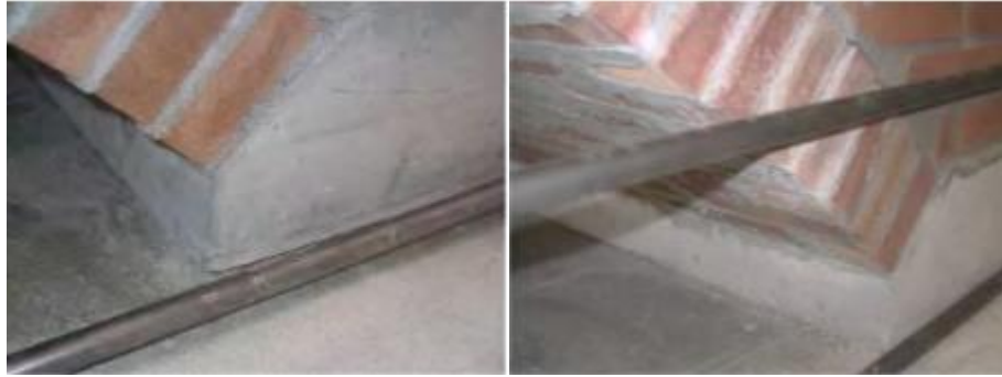
Figure 3-25 risen of the concrete slab and crack at the springing of the ring (Serna, J., 2001).
