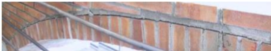
Figure 3-24 large crack between the ring and the spandrel walls (Serna, J., 2001).
