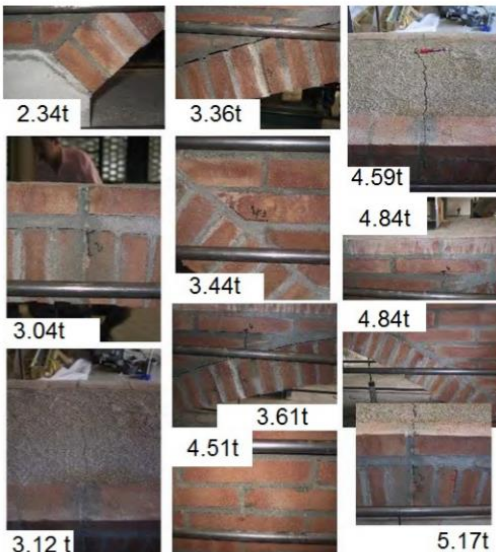
Figure 3-16 cracks before the collapse in the west side (Pereira, R., 2015).
