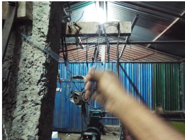
Figure 9. DG operator of Matehari checking the load balance (2014)
