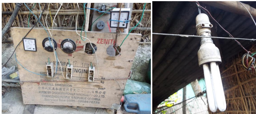
Figure 8. Voltage and amperage board and CFL and lighting point allowed
